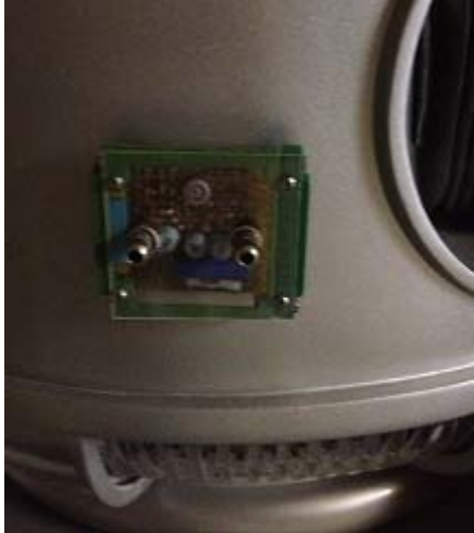
Power Pack Installed
