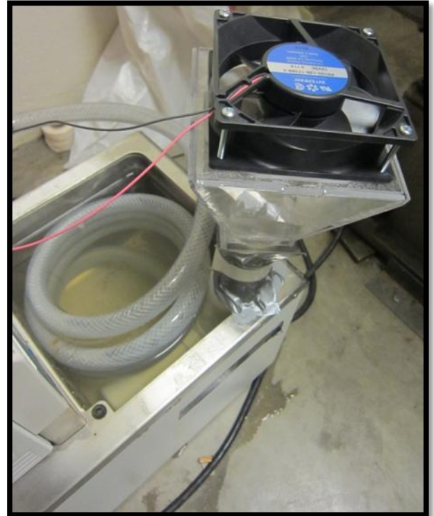
Figure 13: Exit Fan from Condenser
