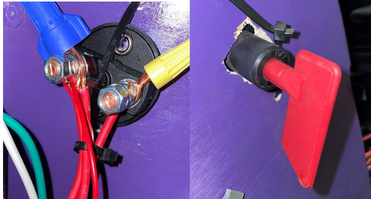
Figure 33: Emergency Disconnect front and back.
